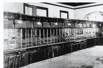
Magnetic parallel multiple telephone switchboard
