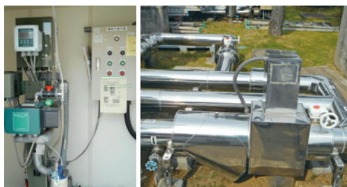
The use of well water was reduced and water quality was maintained by combining a water quality sensor (left) and piping incorporating an automatic switching valve
