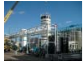
Equipment for the treatment and recycling of waste water at a semiconductor manufacturing site
