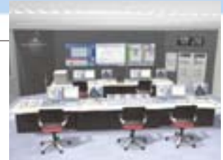
Fire-fighting command and control system
