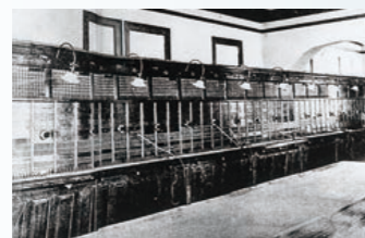
Magnetic parallel multiple telephone switchboard
