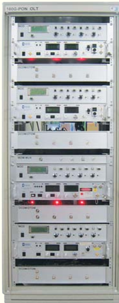
OLT (Optical Line Terminal), the main equipment of this system
