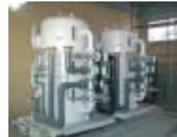
Equipment for producing super-pure water used in semiconductor manufacturing
