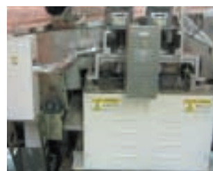
Detection equipment location at flow soldering equipment (solder bath)
