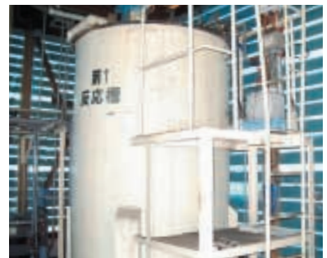
Equipment to treat acid drainage
