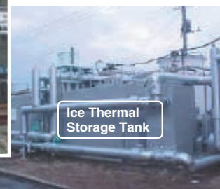
● Installation of "Eco-Ice" (Example from Fiscal 2002)
