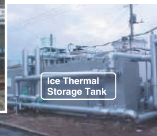
● Installation of "Eco-Ice" (Example from Fiscal 2002)
