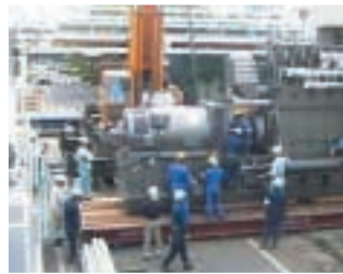
● Installation of a Co-generation System (Example from Fiscal 2000)
