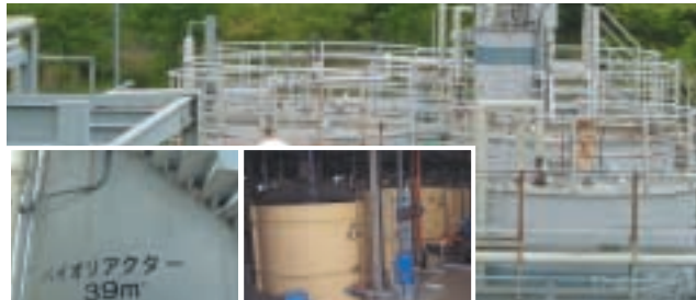
● Bio-recycling System Installed at a Waste Water Treatment Site
