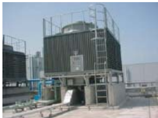
Newly installed cooling tower for free cooling
