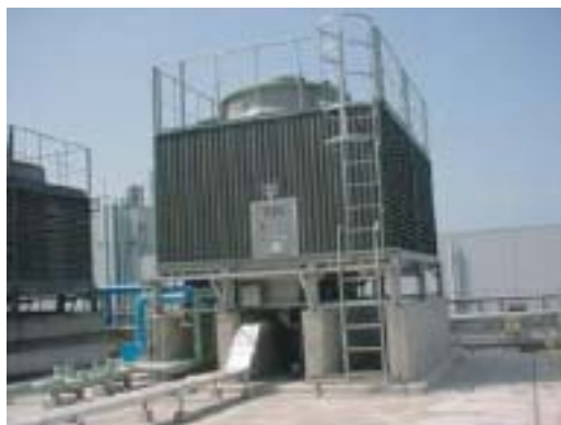
Newly installed cooling tower for free cooling
