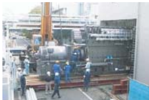
Installation of a co-generation system
