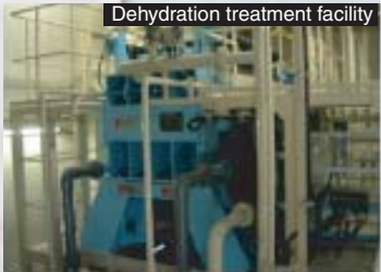
Dehydration treatment facility
