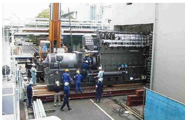
Installation of a Co-generation System
