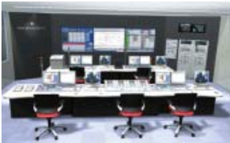
A fire fighting command and control system
