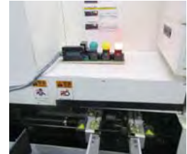
Operators are alerted to equipment operation status by different colored light bulbs
